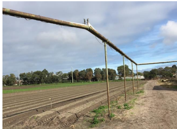
Figure 3: Elevated and uninsulated hot water pipework taking 35°C water from the boiler to the greenhouses
