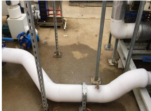
Figure 3: Exposed and uninsulated refrigerant piping
