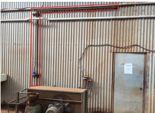
Figure 1: Exposed refrigerant piping running alongside shed
