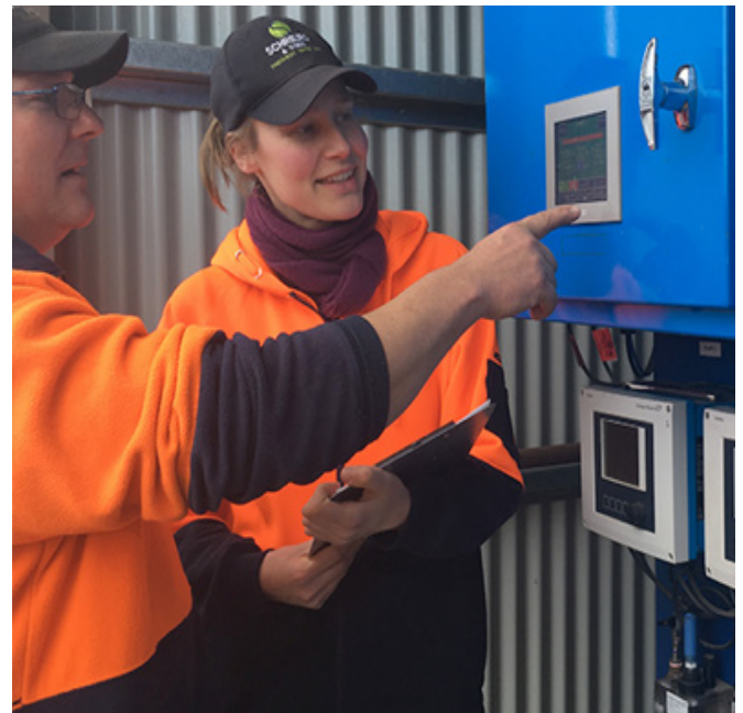
Dr Marie-Astrid Ottenhof, Technical Director Schreurs & Sons with Production Manager Mark Bell, inspecting the Electrolysed Oxidised Water (EOW) sanitation system installed at their packing facility in Clyde, Vic.
